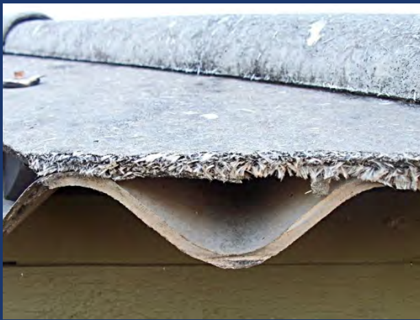
Friable - Roofing Felt
