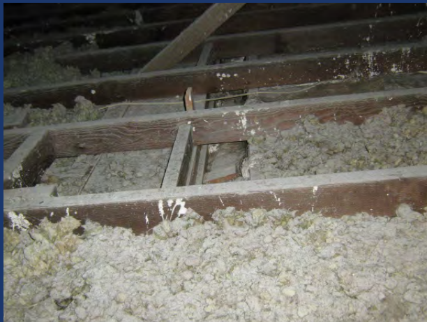
Nonfriable - Loose Insulation
