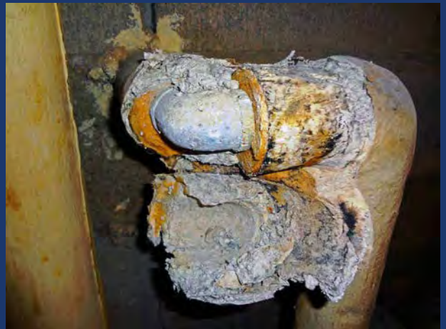
Friable - Pipe Insulation
