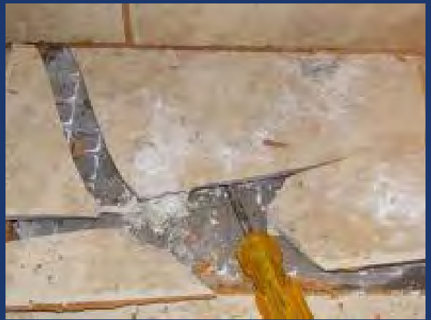
Friable - Vinyl Floor Tiles
